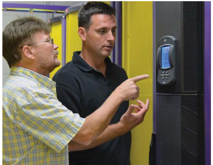
ITCS Operations and Systems manage the Secondary Data Center, located on ECU's Health Sciences Campus.
